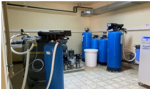
Figure 1: Water treatment system used in the dialysis unit
